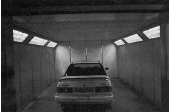
Figure 15.5 Lighting for the spray booth ( Fifth Generation Technology Ltd )
