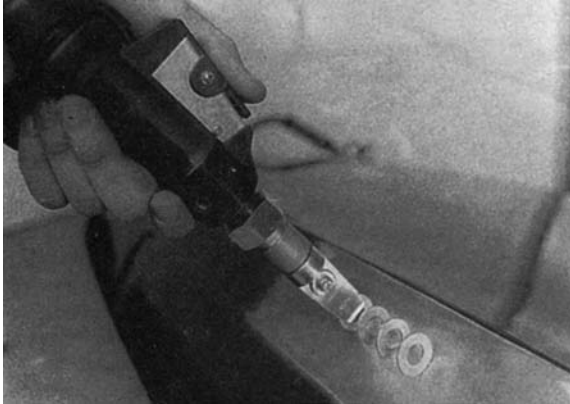
Figure 13.65 Fastening ring washers to the damaged area ready to pull ( Stanners Ltd )
