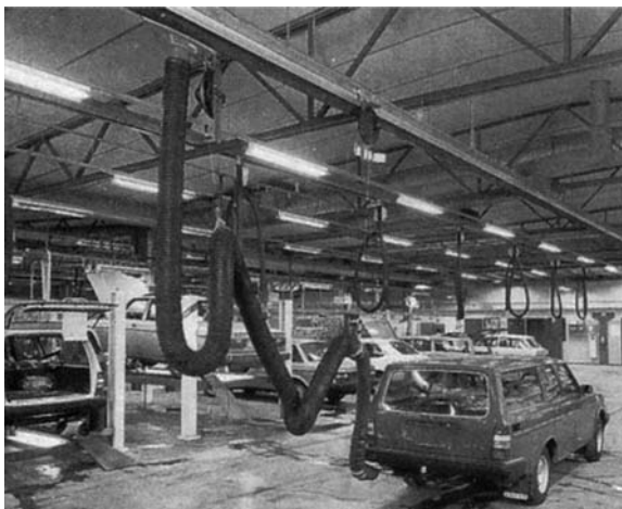
Figure 15.9 Vehicle exhaust extraction using a rail system ( Nederman Ltd )
