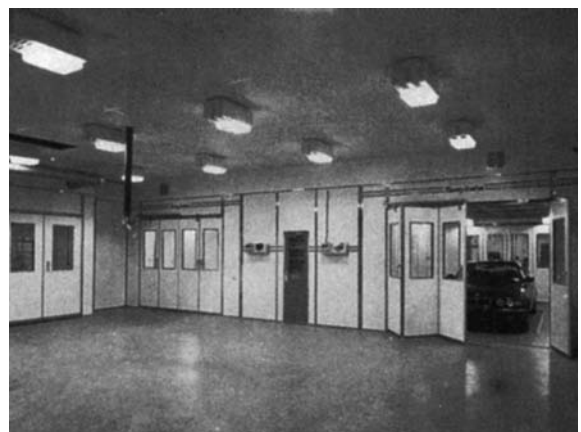
Figure 17.56 Multiple installation showing drive through and paint mix room (integral) between units (Spraybake Ltd)
